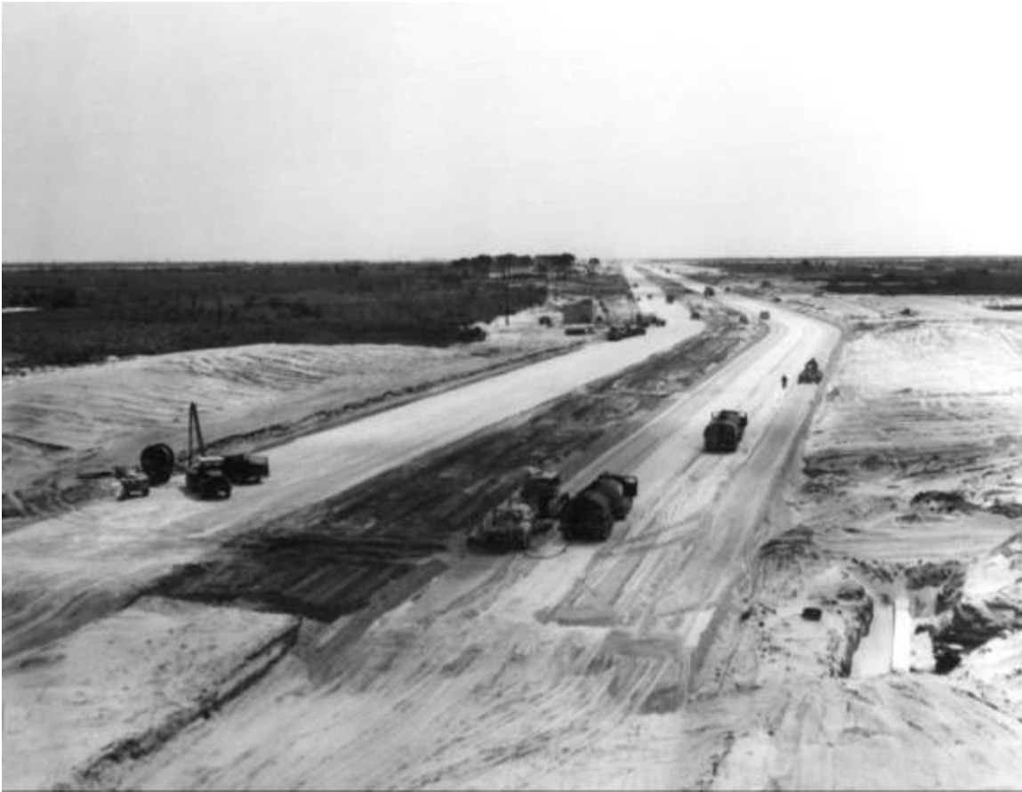
Crawlerway under construction. (3) The communication and instrumentation duct is open in the right foreground (July 1964).
