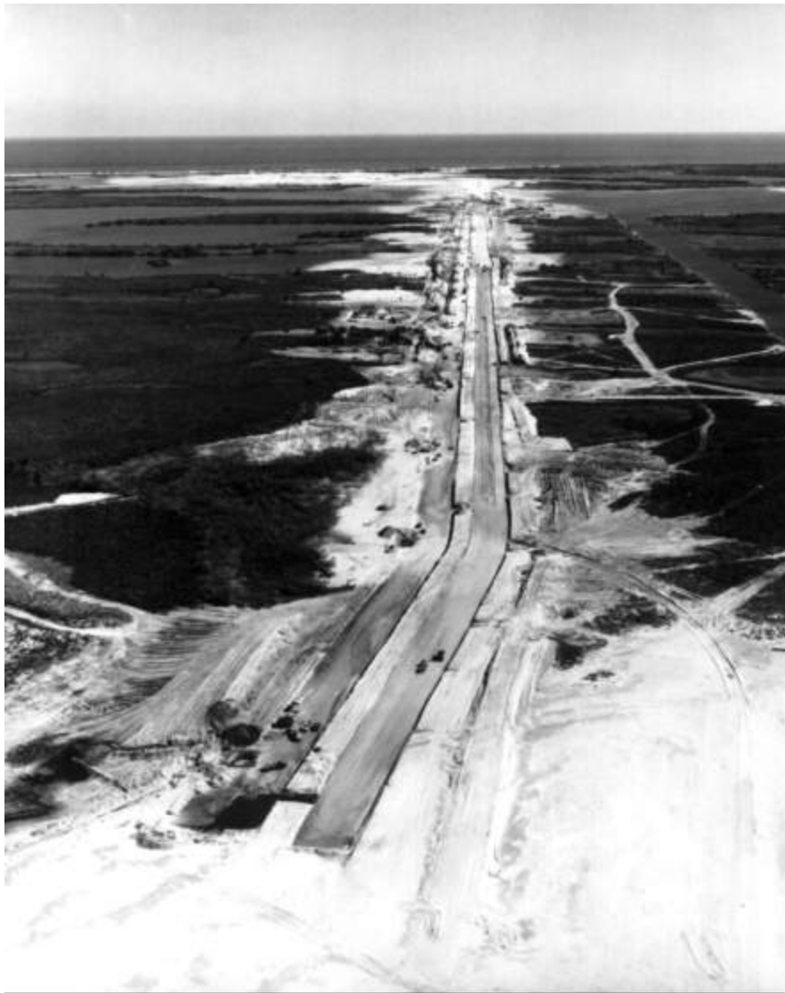
Crawlerway under construction. (1) The terrain was not the best for supporting heavy vehicles (February 1964).
