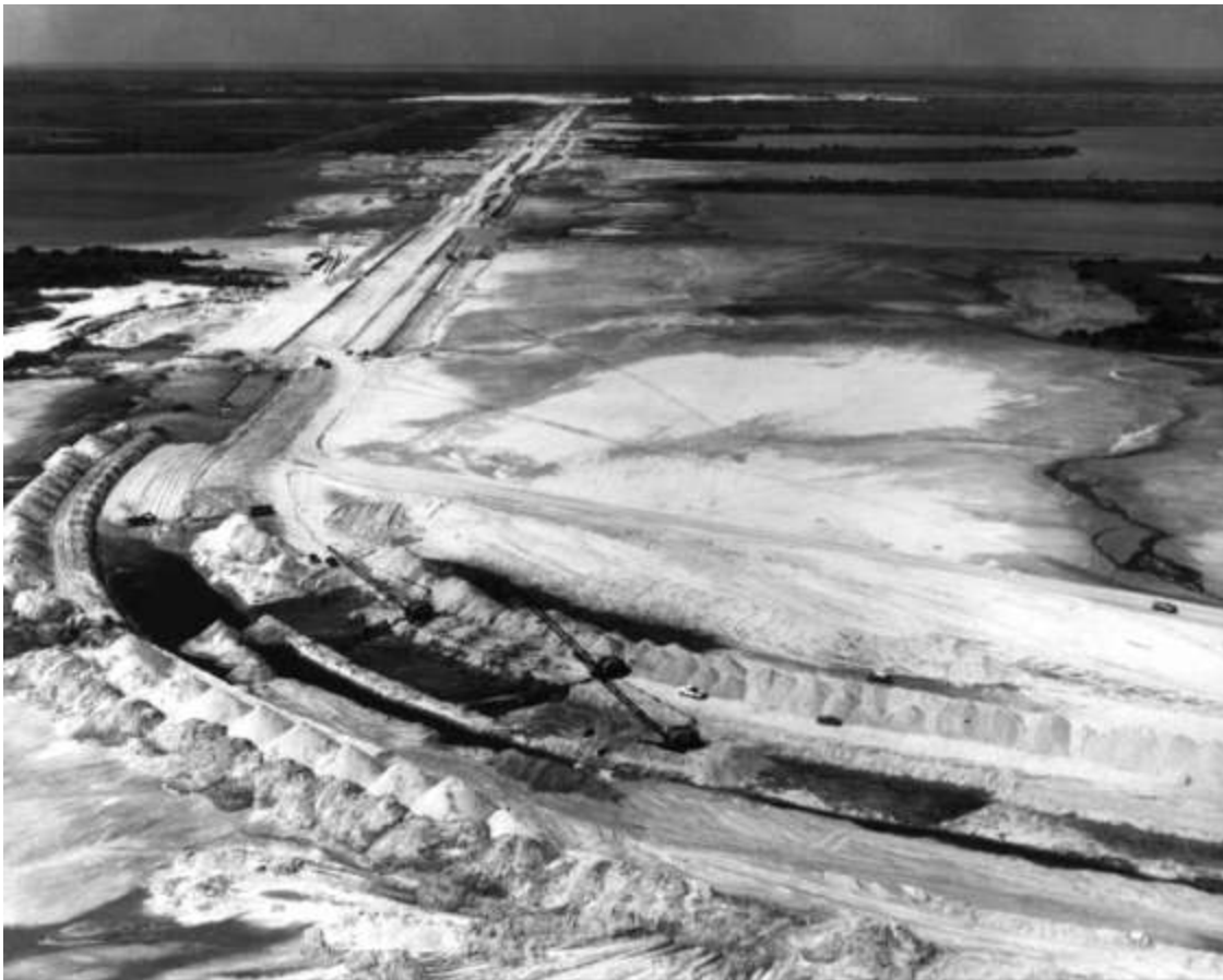
Crawlerway under construction. (2) The site of the assembly building is top, center; pad A is off to the right (April 1964).
